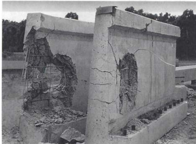
Figure 1.1: Reinforced concrete after EFP impact.(2)
